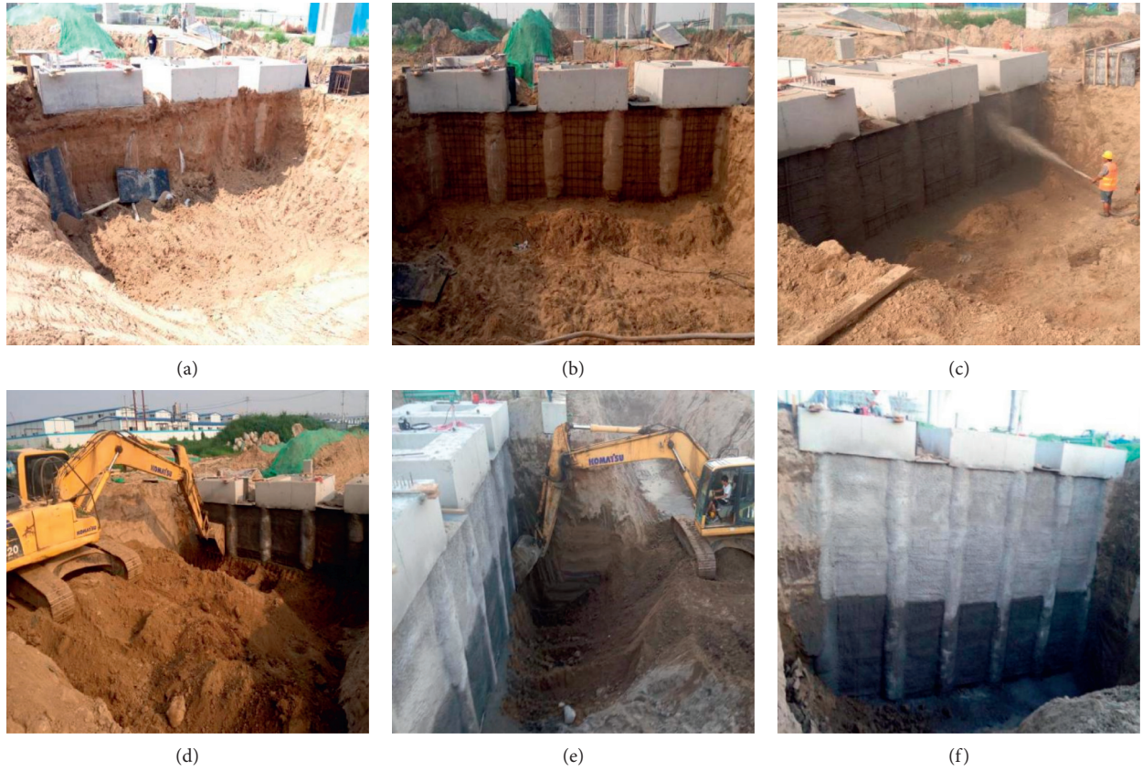
FIGURE 13: Excavation process of foundation pit. (a) Excavation of 2 m. (b) Hanging net between piles. (c) Spraying concrete. (d) Excavation of 4 m. (e) Excavation of 6 m. (f) Excavation of 8 m.
