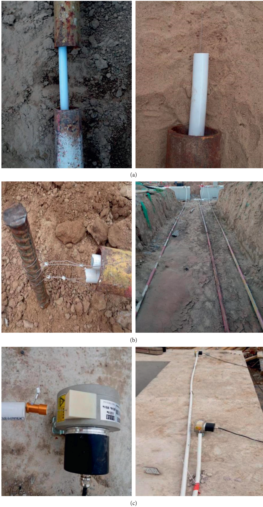
FIGURE 10: Connection diagram of the remote displacement automatic monitoring system. (a) Relative position of the aluminum-plastic tube, iron pipe, and steel strand. (b) Fixed point connection behind the pile. (c) Connection of guyed displacement gauge on the pile top.
