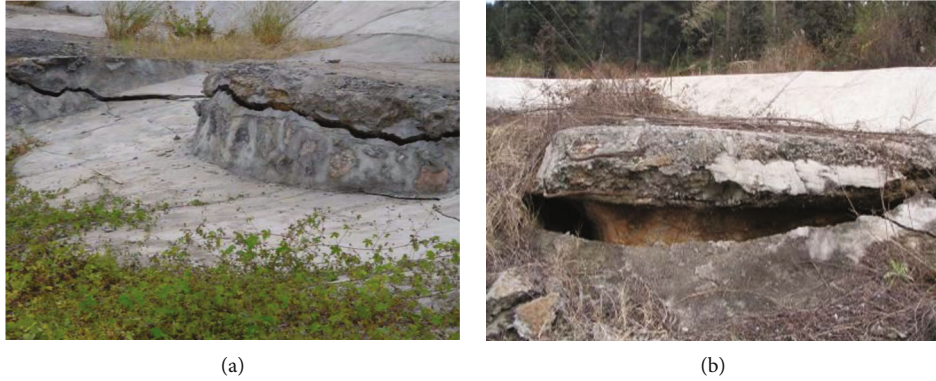
FIGURE 2: (a) Crack behind the piles of the third step in 2003. (b) Crack behind the piles of the third step in 2006.
