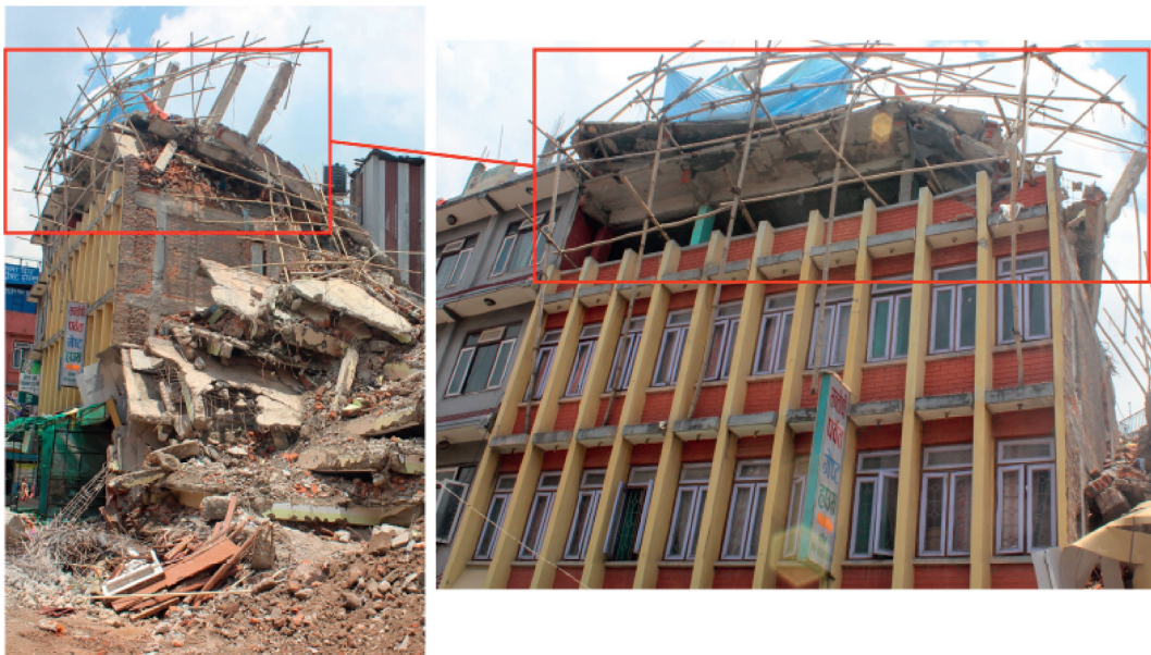
FIGURE 6: Collapsed top story in a soft-story building in Kathmandu by the Gorkha earthquake.
