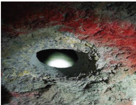
FIGURE 13: Void behind the lining.
