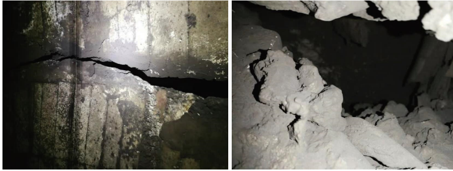
FIGURE 1: Real map of lining diseases of Daheishan Tunnel on Datong to Qinhuangdao Railway.
