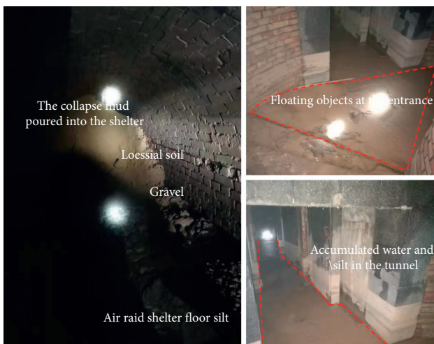
FIGURE 7: Full view of air raid shelter below after collapse.
