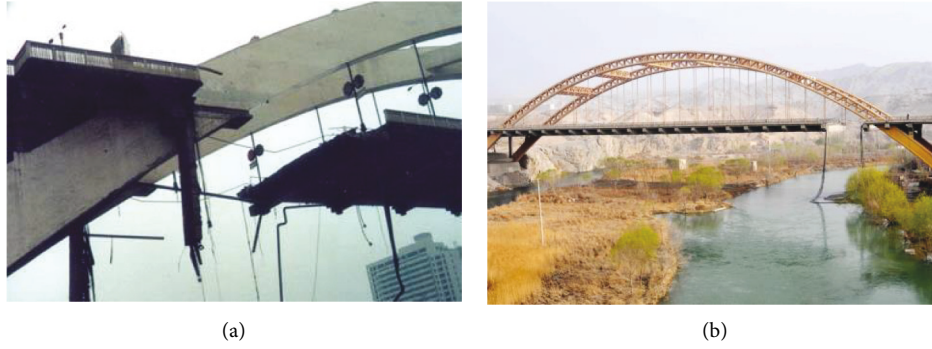
FIGURE 1: Damage forms of different bridge decks.
