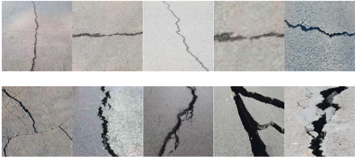
FIGURE 3: The samples of typical crack images.
