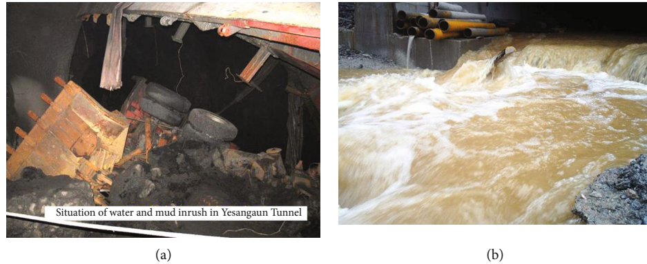
FIGURE 1: Situation of water and mud inrush in the Yesangaun Tunnel [1].
