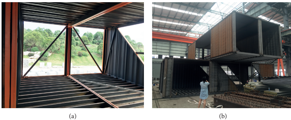
FIGURE 11: Photos of construction site. (a) Site installation of structurally strengthened modules. (b) Factory manufacturing and trial assembly of container building modules.
