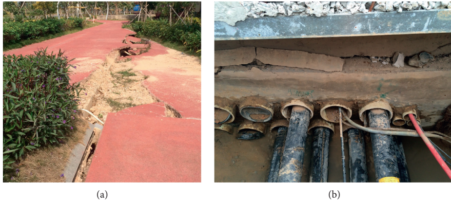
FIGURE 2: Ground subsidence (a) and damage (b) caused by deficiencies in concrete-encased underground electrical duct banks.
