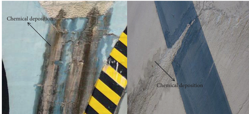
FIGURE 1: Chemical deposition of seepage water.
