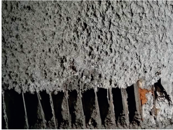
FIGURE 18: Primary support cracking (scheme III).
