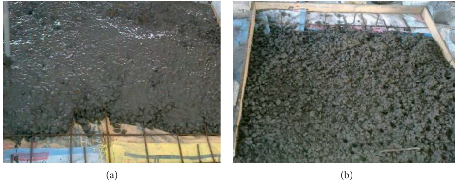
FIGURE 3: A view of making of waste paper concrete slab. (a) Conventional mix. (b) Glass-fiber reinforced mix.
