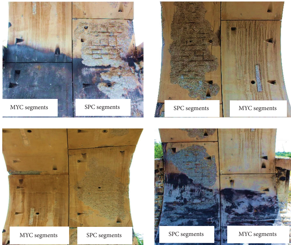
FIGURE 9: Spalling at different locations of SPC and MYC segments.
