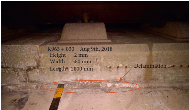
FIGURE 2: Example of delamination of CRTS II SBTS from the on-site survey of the Beijing-Shanghai HSR.
