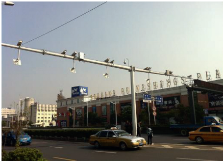
FIGURE 2: Picture of the actual installation.
