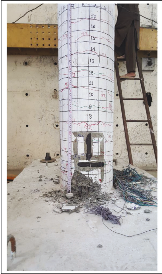
FIGURE 3: Damaged column, cracks, and spalling of concrete.
