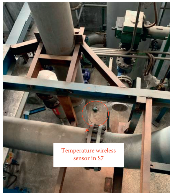
FIGURE 18: Display of the wireless temperature sensor at the S7 position on the first floor of the gantry.
