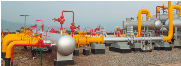
FIGURE 11: The inlet pipelines after modifications.
