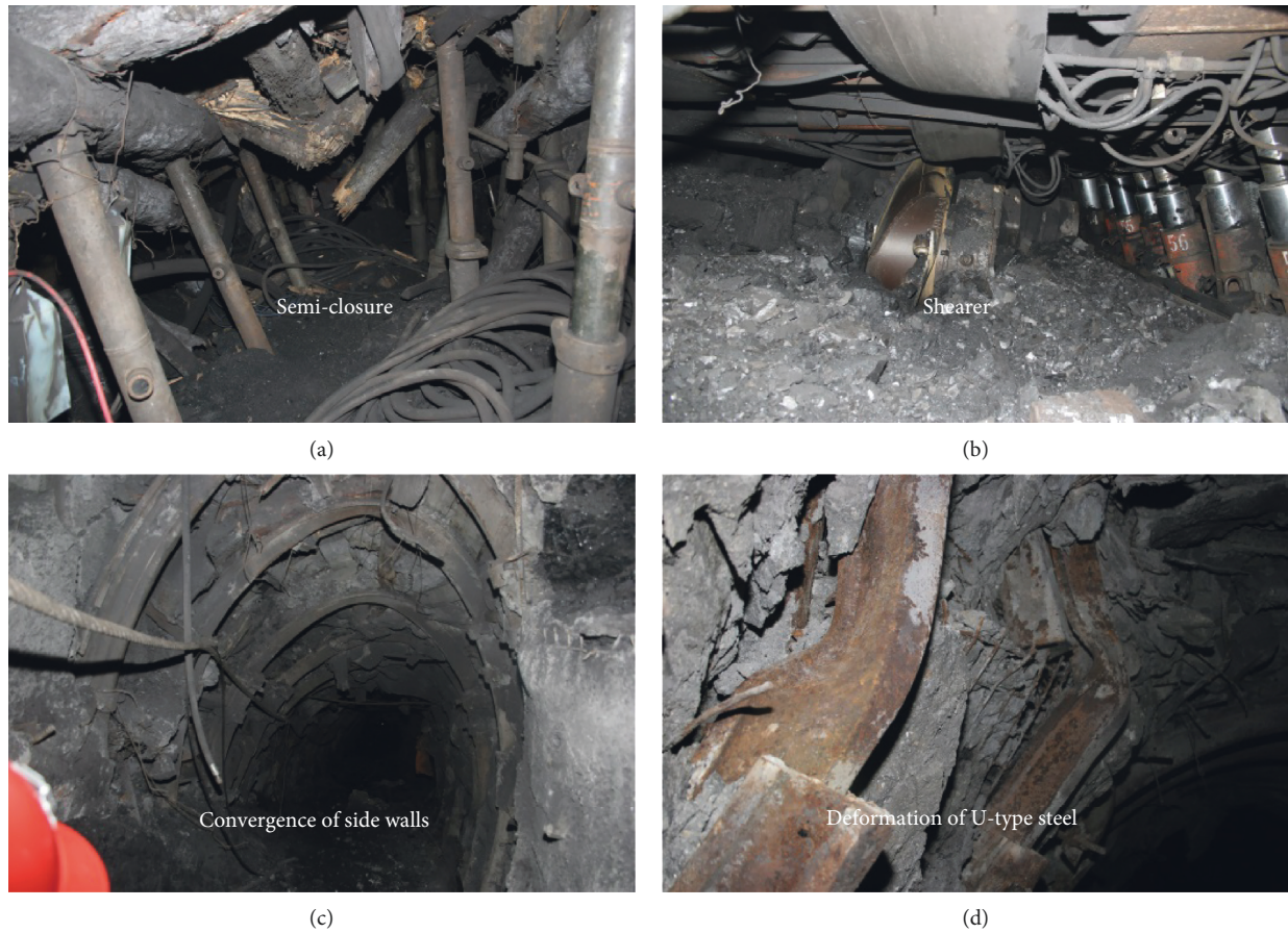
FIGURE 2: Photos of rockburst damage in Xing'an Coal Mine, roof subsidence and floor heave (a), coalface damage (b), convergence of two side walls (c), and damage of U-type steel (d).
