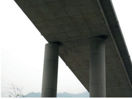
FIGURE 1: Unseating of Baihua Bridge caused the Wenchuan earthquake.
