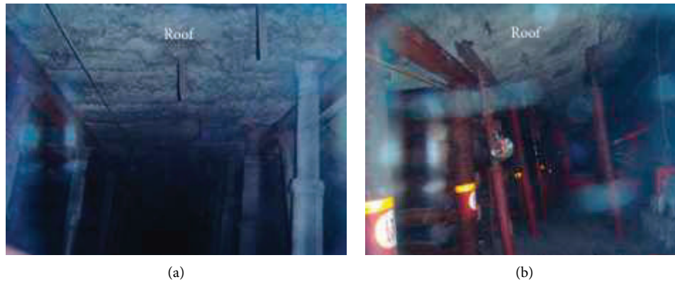
FIGURE 13: Roof form of the gob-side entry retaining in the reuse period. (a) Roof form in section 1; (b) roof form in section 2.
