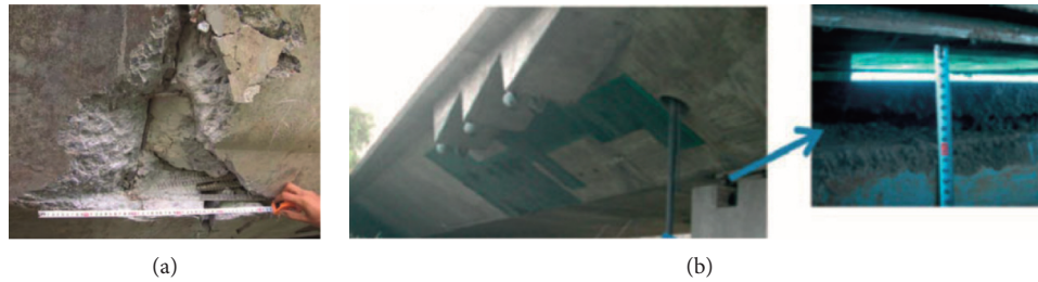
FIGURE 7: Damage patterns of the Tianjin Yonghe Bridge. (a) Cracks at the closure segment at both side spans. (b) Damaged concrete piers of the bridge. Adapted from “Structural health monitoring of a cable-stayed bridge with Bayesian neural networks” by Stefania Arangio & Franco Bontempi (2015), Structure and Infrastructure Engineering, 11 : 4, 575–587, reprinted by permission of Taylor & Francis Ltd.
