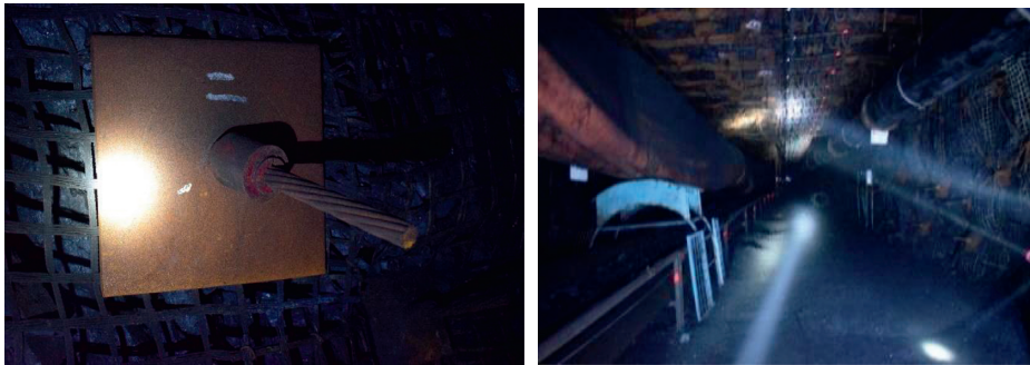
FIGURE 16: Deformation of 600 m side of return airway.
