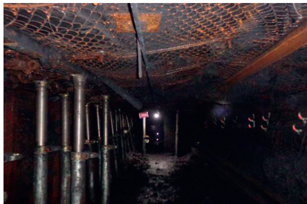
FIGURE 13: Effect of retaining the entry in the track crossheading of the 2103 working face.
