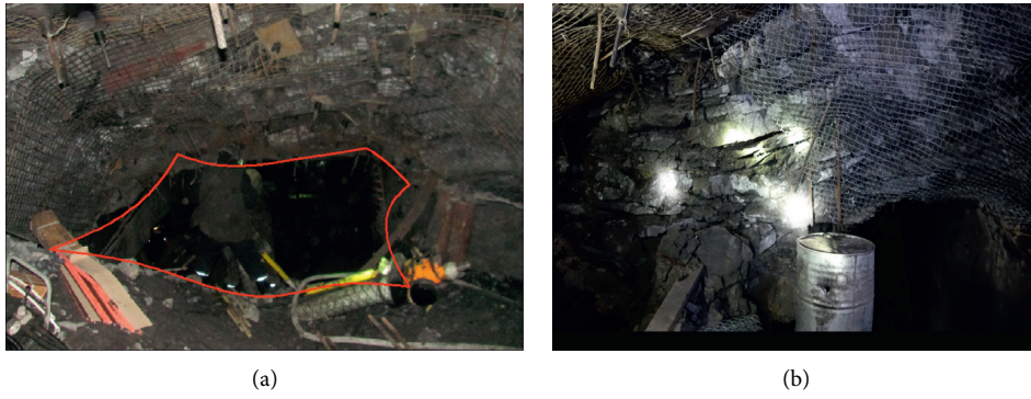
FIGURE 18: Deformation and failure of roadway surrounding rock. (a) Deformation and failure. (b) Layered joints.
