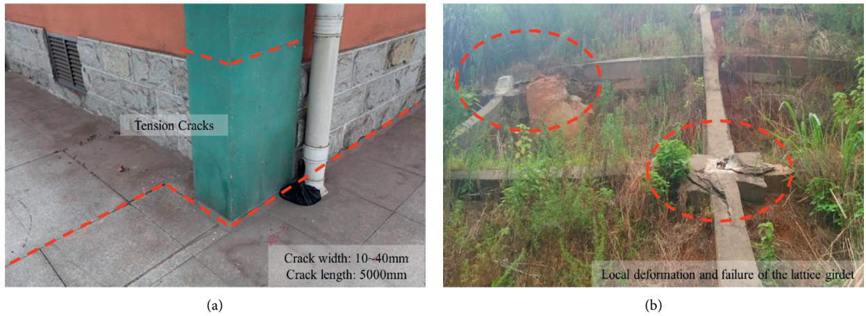
FIGURE 2: (a) Tension cracks in the exterior wall of museum and (b) local deformation and failure of lattice girder on the east-side slope of north open-pit mine [32].
