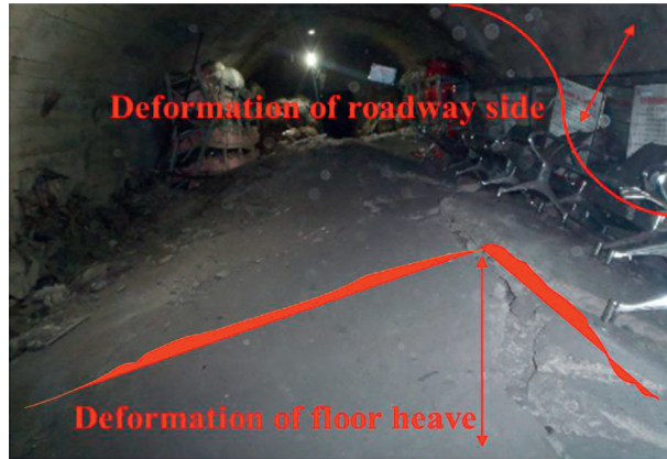
FIGURE 1: Deformation and failure of the roadway.
