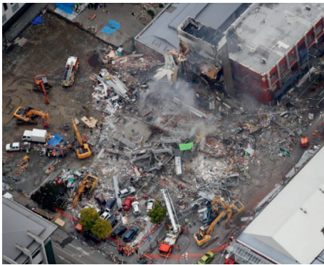
FIGURE 5: Rescue workers in a collapsed building after the earthquake in Christchurch, New Zealand, February 23, 2011.
