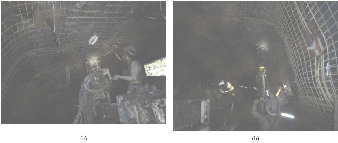
FIGURE 18: Site anchor bolt construction. (a) Hydraulic bolting rig in action. (b) Hand-held pneumatic bolt drill in action.
