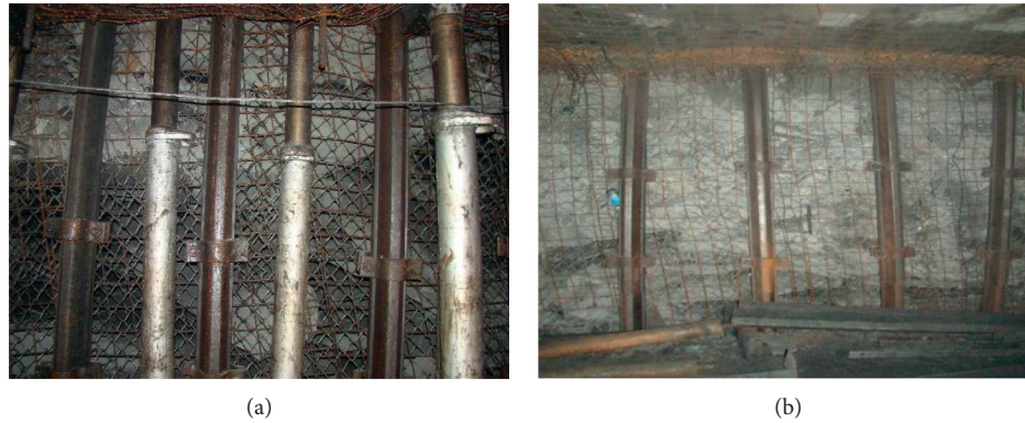
FIGURE 10: Effect of blocking gangue. (a) Blocking-gangue support installation. (b) Hydraulic prop remove.
