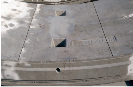
FIGURE 1: The defective shield tunnel segment.
