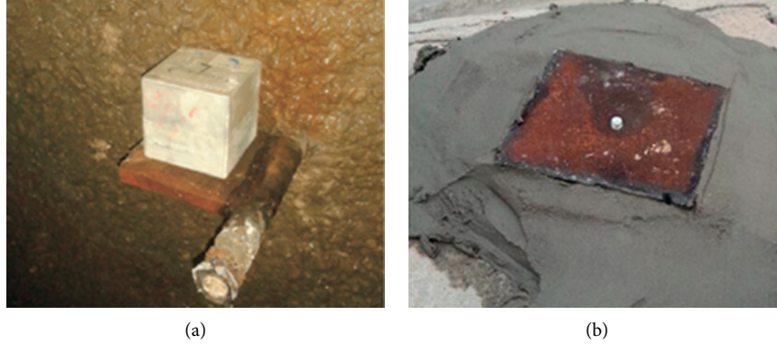
FIGURE 5: Photographs of installed sensors. (a) Measuring point in the tunnel. (b) Measuring point on the slope surface.
