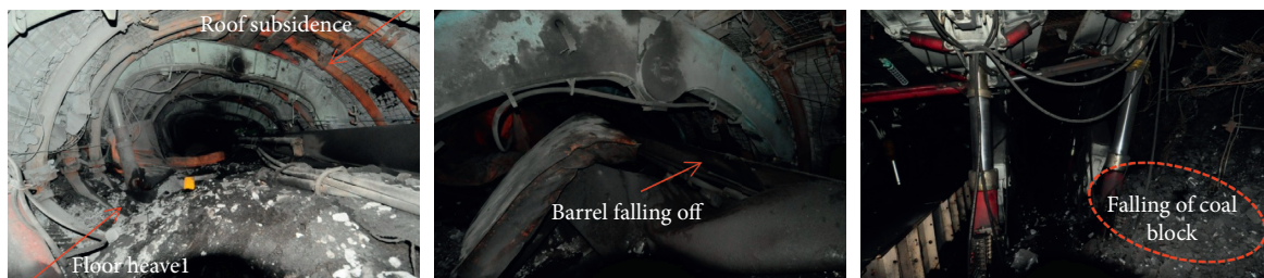
FIGURE 8: Scene photos of roadway rock burst accident in Yuejin mine.
