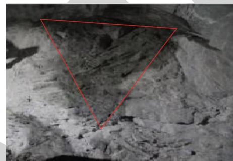
FIGURE 27: Destruction of the deep and large structural plane in K0 + 545 m of the tailrace surge chamber pilot hole.
