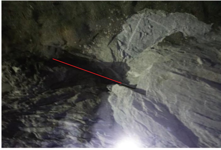
FIGURE 28: Wedge cavity of arch shoulder in K0 + 540 m of the tailrace surge chamber pilot hole downstream.
