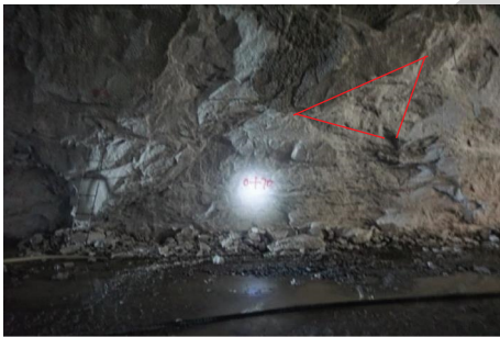
FIGURE 25: Fault slip-type rockburst on the upstream side of the pilot tunnel in K0 + 70 m of the main transformer chamber.
