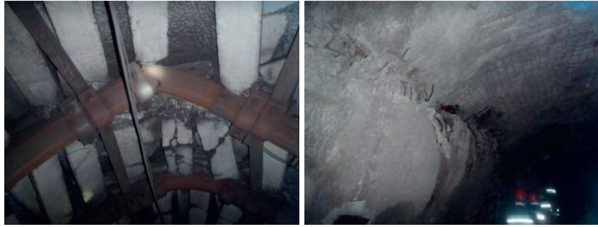
FIGURE 3: Deformation of the main roadway.
