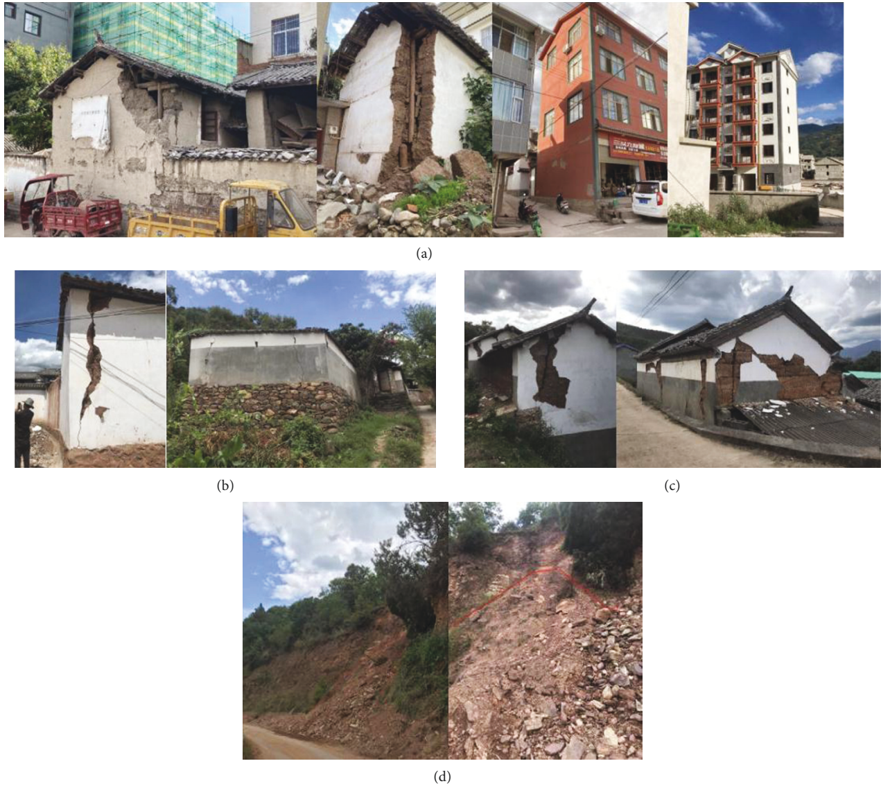
FIGURE 5: Typical seismic damage phenomenon in Yangbi Ms 6.4 earthquake. (a) Damaged buildings in Xiajie Village, Yangbi County. (b) Damaged buildings in Huaian Village. (c) Damaged buildings in Shahe Village. (d) Small landslides in Shahe Village.
