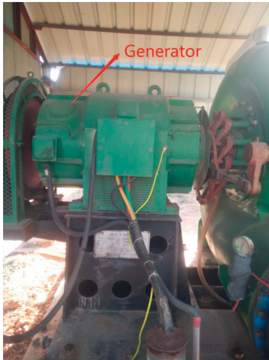
FIGURE 2: Measuring point layout of the generator.
