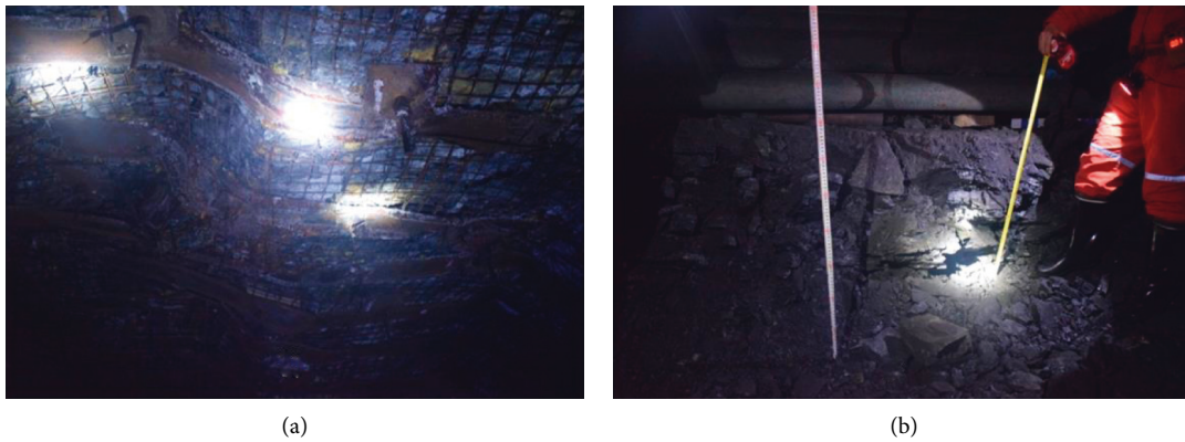
FIGURE 2: Deformation and failure characteristics of similar roadway, i.e., return air roadway 4103. (a) Roof sinking. (b) Floor heaving.
