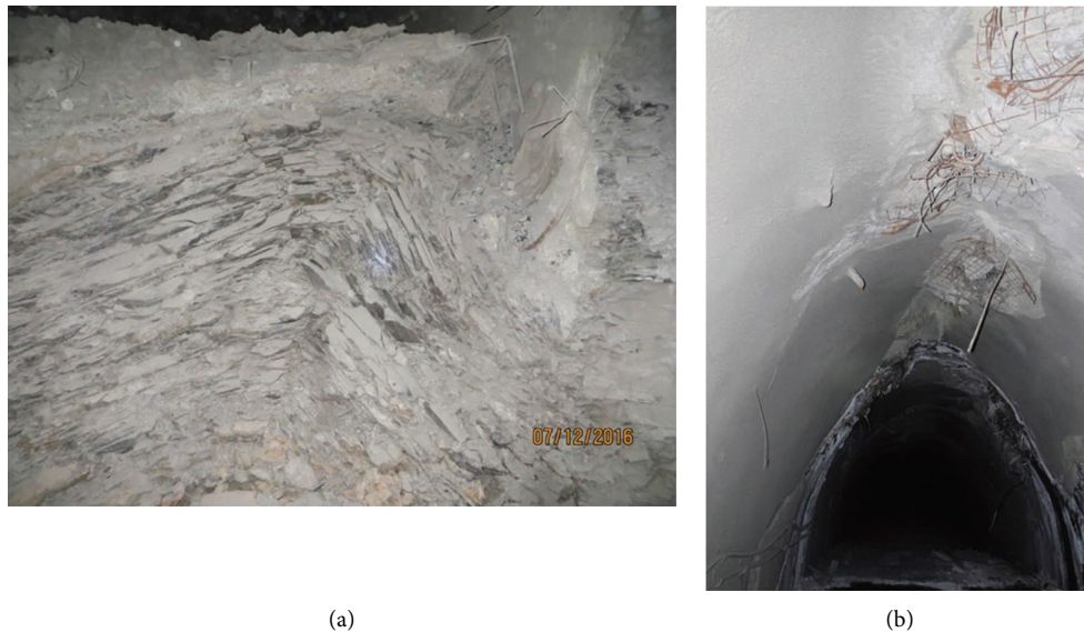
FIGURE 2: Photo of tunnel deformation in Hetaoyu coal mine. (a) Auxiliary transportation lane. (b) Auxiliary transportation stone gate.
