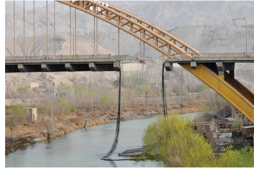
FIGURE 1: Bridge deck collapse due to boom breakage.
