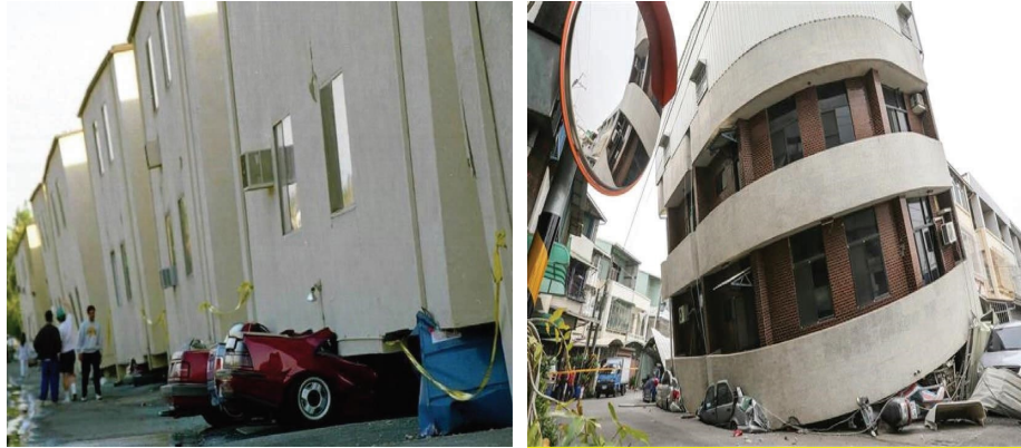
FIGURE 1: Damage caused by soft-story irregularities in a past earthquake.
