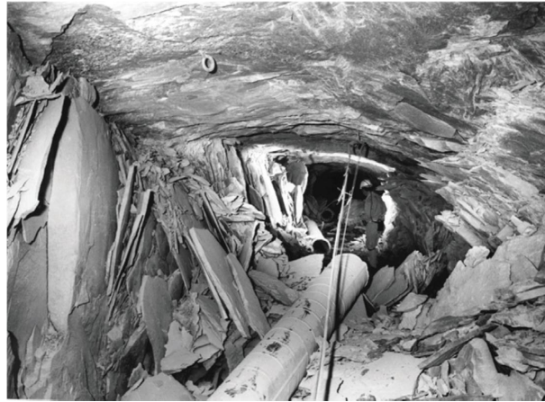
FIGURE 9: Marble rock roadway failure diagram [35].
