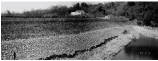
FIGURE 2: The sliding failure zone in Kitayama dam caused by Kobe 1995 earthquake.
