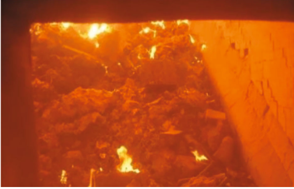
FIGURE 1: Municipal solid waste incineration.
