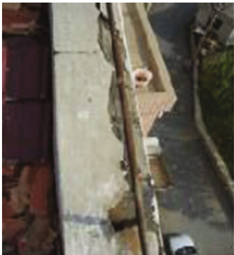
FIGURE 5: Roof parapet damage.
