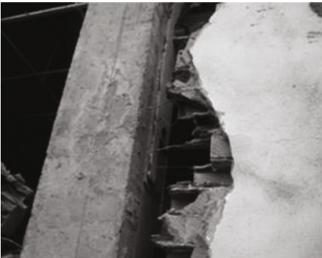
FIGURE 3: Wall column connection failure.
